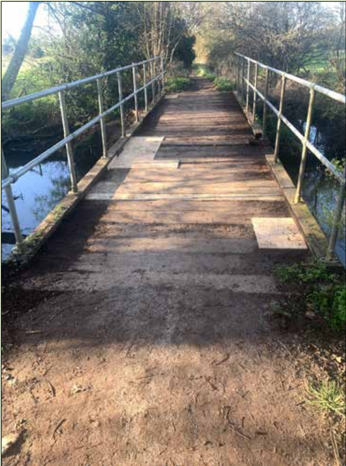
The patched-up bridge.
