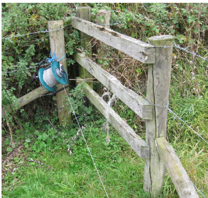
Spot the faults on this 'stile'.
